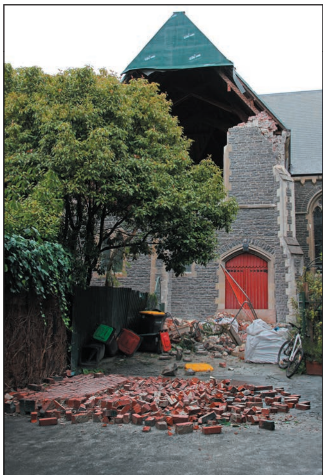
Figure 3. The manager's garden with grey mud expelled by the liquefaction in the foreground, and debris from the two collapsed walls of his neighbours.
