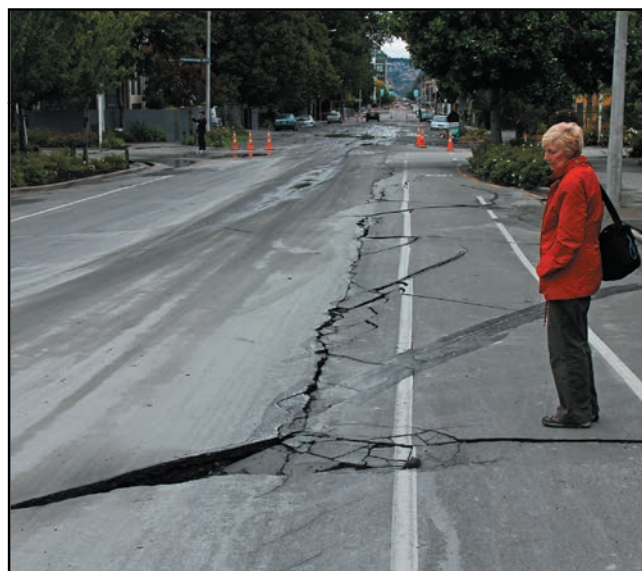
Figure 8. A cracked road in the city centre.
