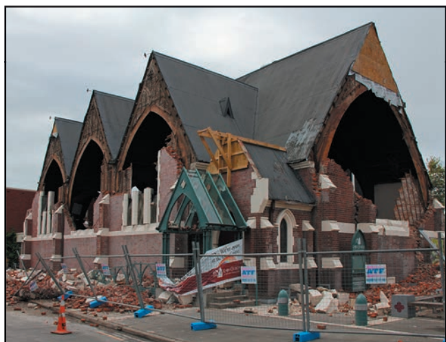
Figure 6. A church that was damaged by both the earthquakes that struck Christchurch, in February of 2011 and in the previous September.
